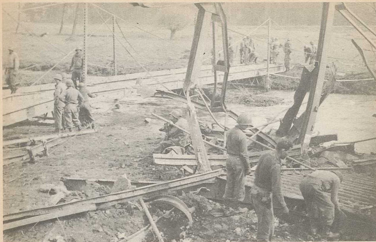
Another river – another bridge to build. It seemed there was always one more.
